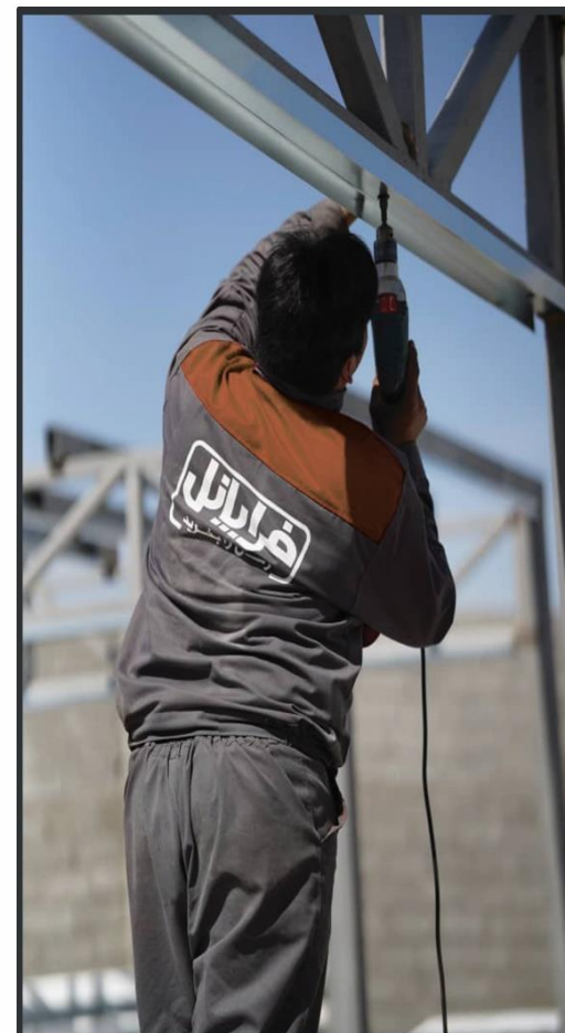
Installing the runner under the ceiling exactly parallel to the floor runner 2
